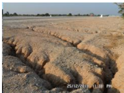
Fig. 3: Channel and Piping Erosion
