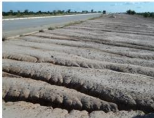
Fig. 2: Channel and Piping Erosion
