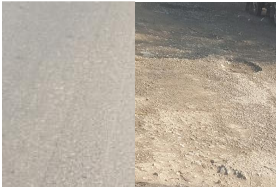
Figure 1.1 (a) shows good condition while (b) shows failed condition scenario
